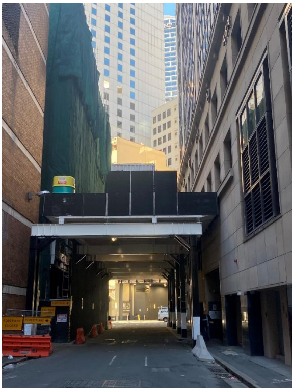
Figure 4: Existing hoarding and site sheds viewed from Dalley Street looking east. The construction site for which this hoarding is for is on the left and the ASX building is on the right.
