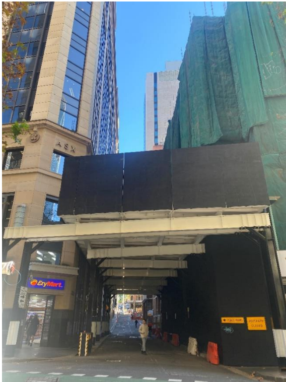
Figure 3: Existing approved hoarding viewed from Pitt Street looking west. The construction site for which this hoarding is for is on the right and the ASX building is on the left.
